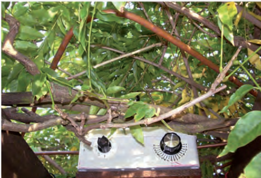
Fig. 4: The tuner and counterpoise at the top of a pergola, and hidden in a Wisteria!
